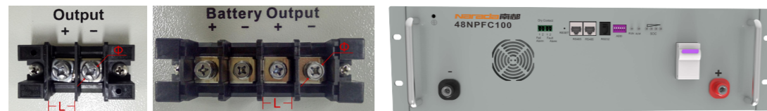
Fig.1-2 Battery Output Terminal
